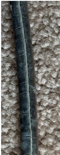
Right: Black coax stands up better to UV but will still crack with age.
