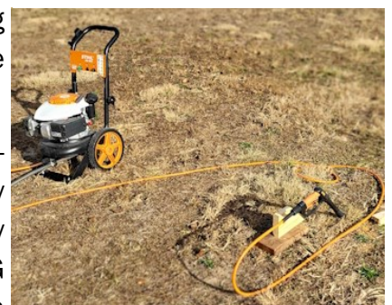
A pressure washer was used to drill a pilot hole and loosen the soil. Yes, it covered me in mud.
