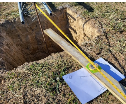
Measurements were made to set the tower legs at compass directions 0 deg (North), 120 deg, and 240 deg.
