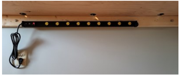
Power strips were installed under the desk.
