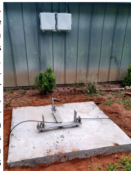
Two waterproof utility boxes were mounted on the outside of the shack, near the base of the tower
