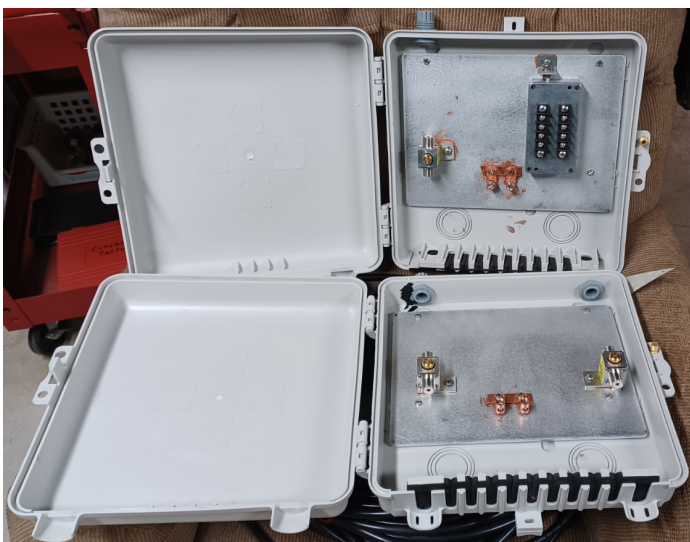
Below: The coax and rotator cable lightning arrestors will be mounted in weatherproof boxes.
