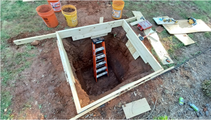
A concrete form was built after digging the bottom of the hole out by hand.
