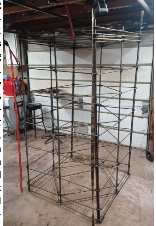
The completed rebar cage is ready to lower into the hole. US Tower provided very specific instructions on the dimensions, shape, and type of rebar required.
