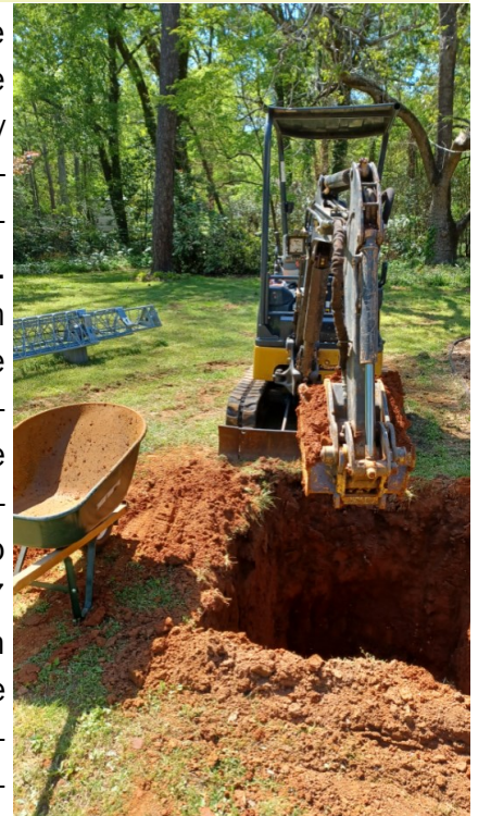
The excavator was only able to reach about 6 ft. below the surface.
