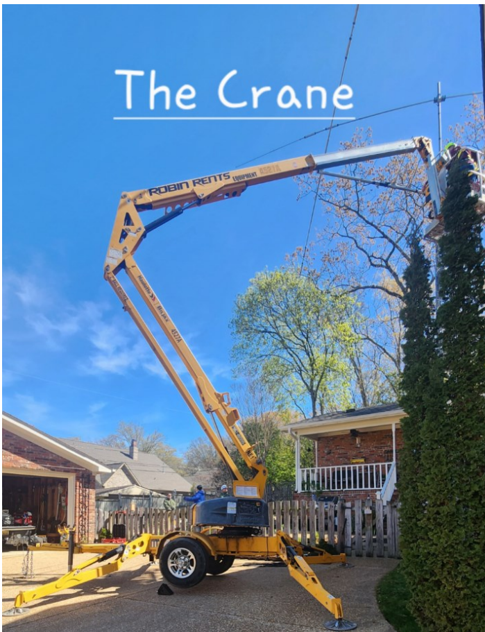
The 51-ft aerial lift made working on the antennas much more manageable.
